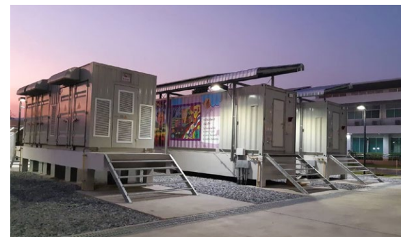
Picture depicts Battery Energy Storage System, size 3 megawatts/ 2.2 MWh of Microgrid Development Project at Mae Sariang District, Mae Hong Son Province, of the Provincial Electricity Authority.
